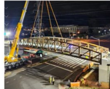
W & OD Pedestrian Bridge over Wiehle Avenue (at Sunset Hills Road), Reston
